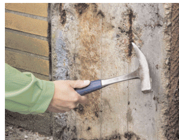
Clearly visible: Concrete maintenance is due here
