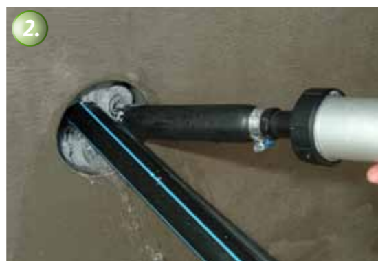
The material is pressed into place between the cable and the wall with the KÖSTER Special Caulking Gun, immediately and permanently stopping the water flow.
