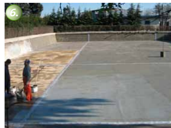
The tiles are applied on top of the waterproofing with common tile adhesive.
