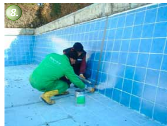
The horizontal joints are waterproofed with KÖSTER Joint Sealant FS-H. The vertical joints were waterproofed with the putty-like KÖSTER Joint Sealant FS-V.
