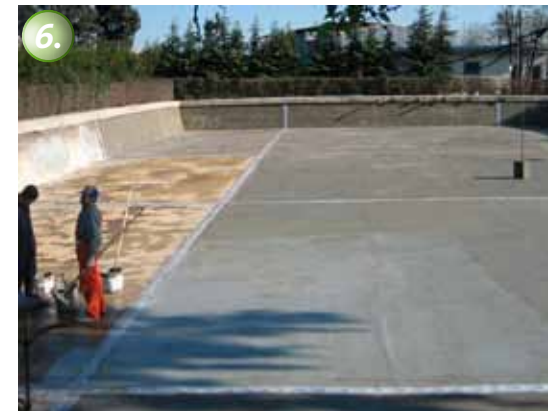
6. The tiles are applied on top of the waterproofing with common tile adhesive.
