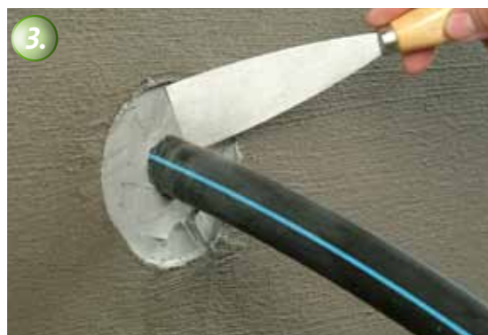
To protect the waterproofing the area is smoothed and protected with KÖSTER KB-Fix 5.
