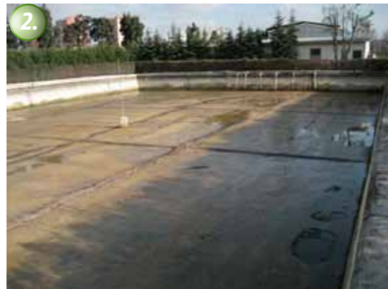
The surface is cleaned down to a solid and stable base material. The substrate must be clean, solid, and free from adhesion inhibiting materials.
