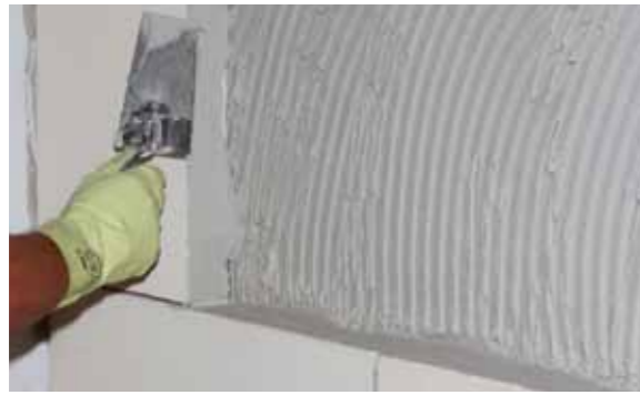
A bead of KÖSTER Hydrosilicate Adhesive SK is applied along edges of the boards to make sure that the joints are fully filled.
