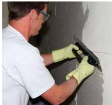
After the KÖSTER Hydrosilicate boards have been applied the surface can be sanded smooth. Subsequently the whole area is plastered with a layer of KÖSTER Hydrosilicate Adhesive SK in a
