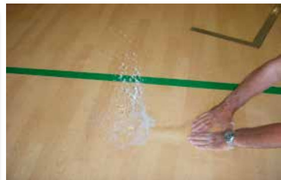
...containing high pH corrosive liquid
