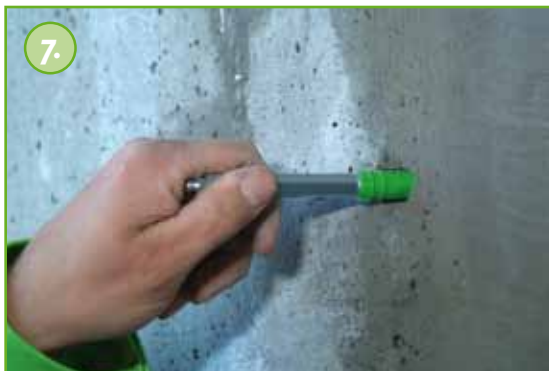
Install KÖSTER Superpackers in the boreholes leaving about every third borehole open.
