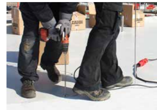
The KÖSTER TPO Membrane is mechanically fastened by attaching the disc anchors to the substructure. In this case, trapezoidal sheet metal.
