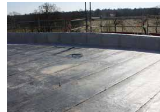
Preparation of a roof surface. A vapor barrier is used as the basis for further installation.
