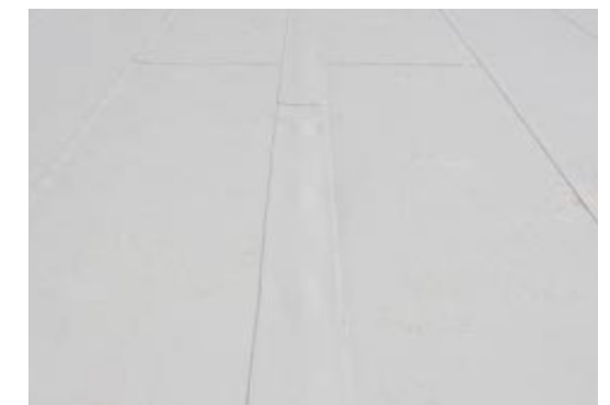
Additional mechanical fastening centered in the membrane may be necessary in order to protect the TPO membrane against high loads.
